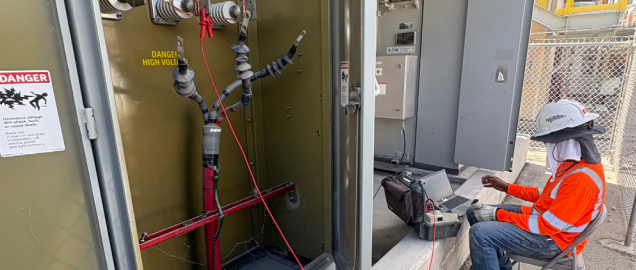
GENERAL ELECTRICAL EQUIPMENT INSTALLATION, MAINTENANCE & TESTING
