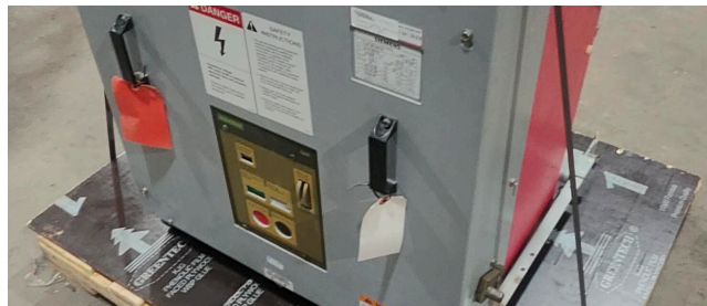
CIRCUIT BREAKER SERVICES
